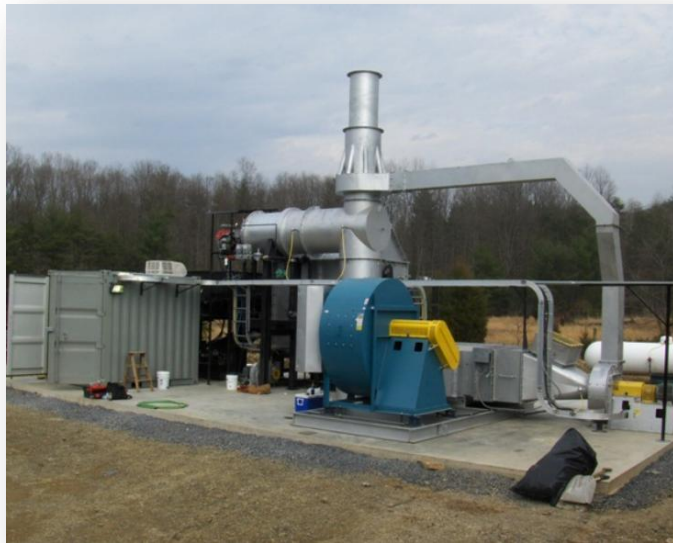
Gasifier at Frye Poultry Farm, West Virginia, USA
